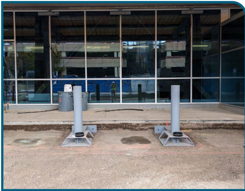
Bollards Designed to Protect the Terminal Building and the Underground Utilities
